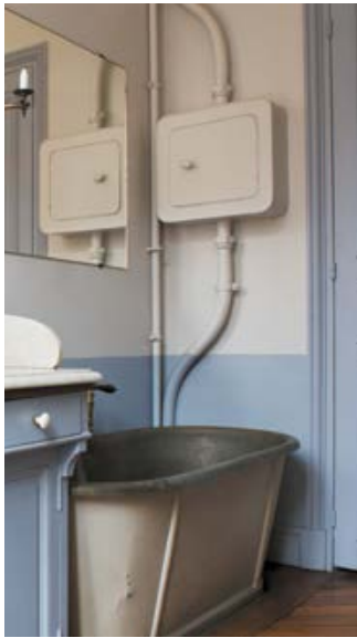
With a bathtub, hot and cold water and a heated towel cabinet, the bathroom boasted a level of comfort rarely seen at this time.
